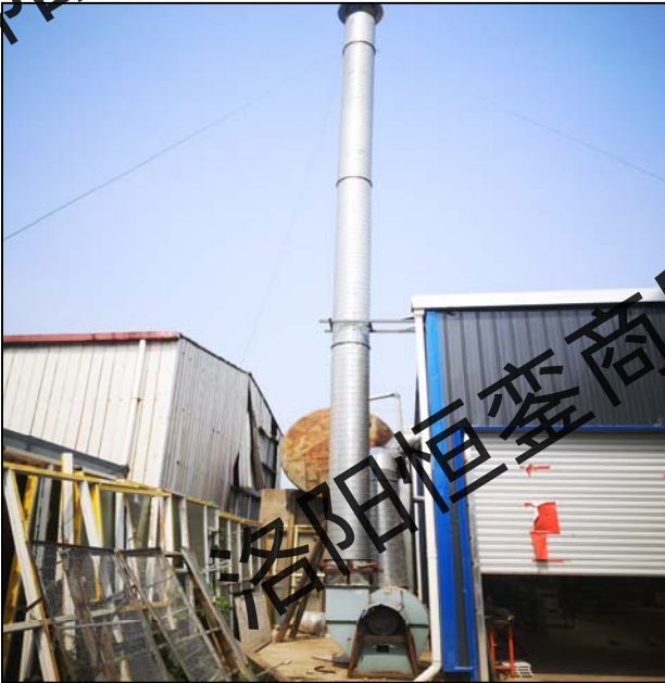
袋式除尘器+15m 排气筒
