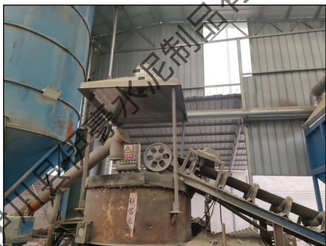
搅拌机收尘措施集气罩
