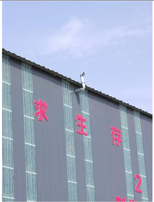
焊接烟尘除尘器排气筒
